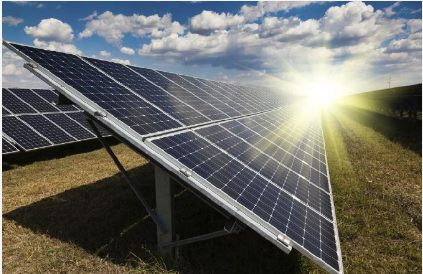
Figure S2: Solar plus energy storage project in North Carolina
